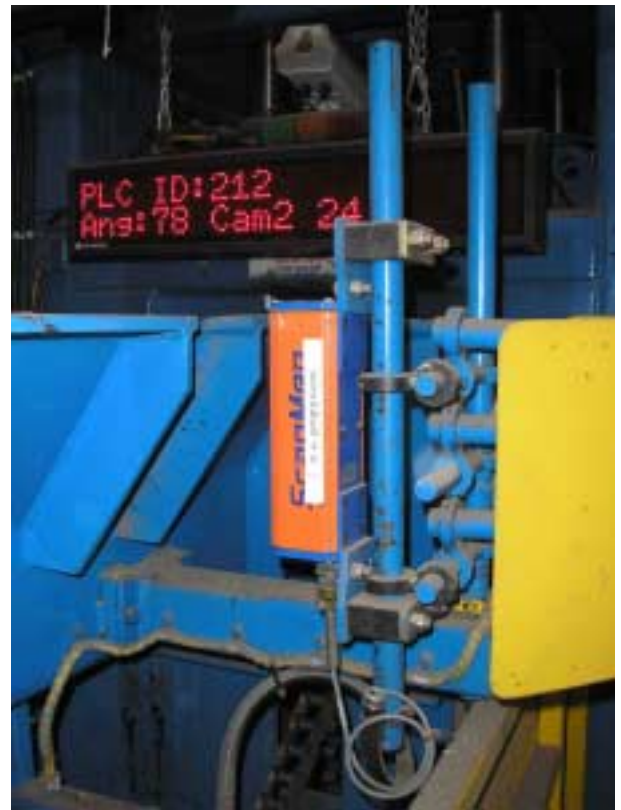
V-flight conveyor photocell feeding USNR canter/circle quad with Curve-sawing VSA
