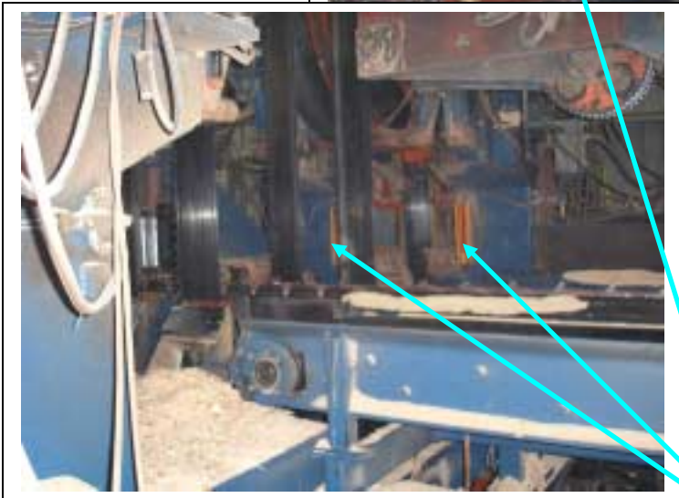
ScanMags before and after Quad Bands at Simpson Timber's mill in Tacoma – handles dust just fine!
